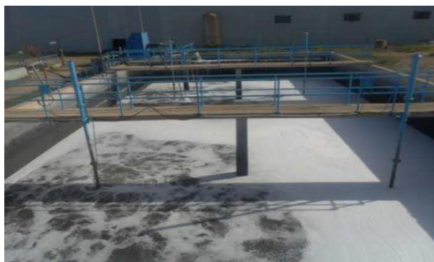
Figure 2. Photo of mixing and equalization basin N ° 1.
