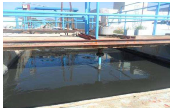
Figure 3. Mixing and neutralization basin N ° 2.
