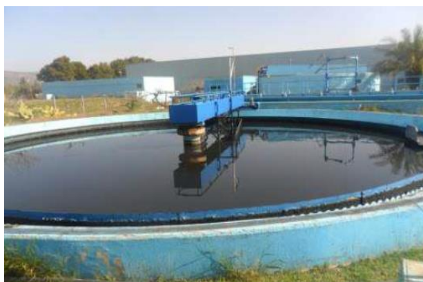
Figure 6a. Final clarification basin.
