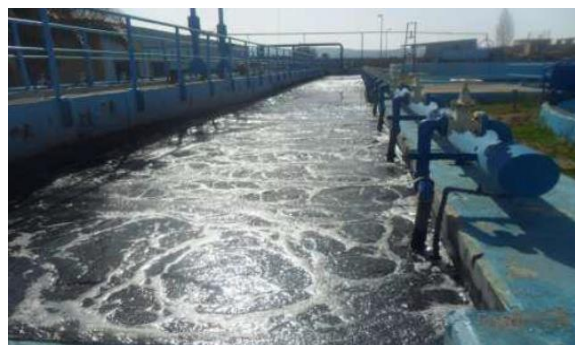
Figure 5. Biological basin (aeration basin).
