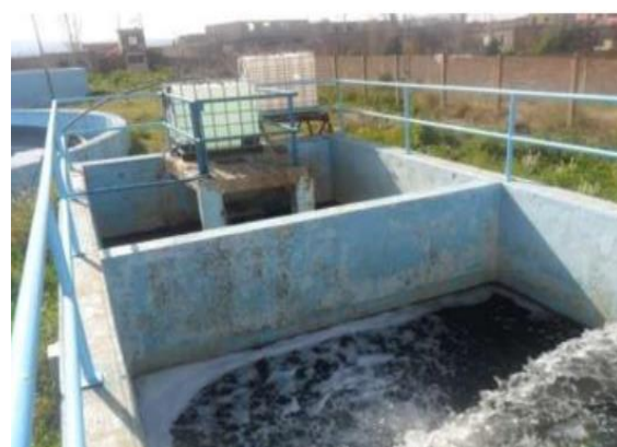
Figure 6b. Post chlorination basin.
