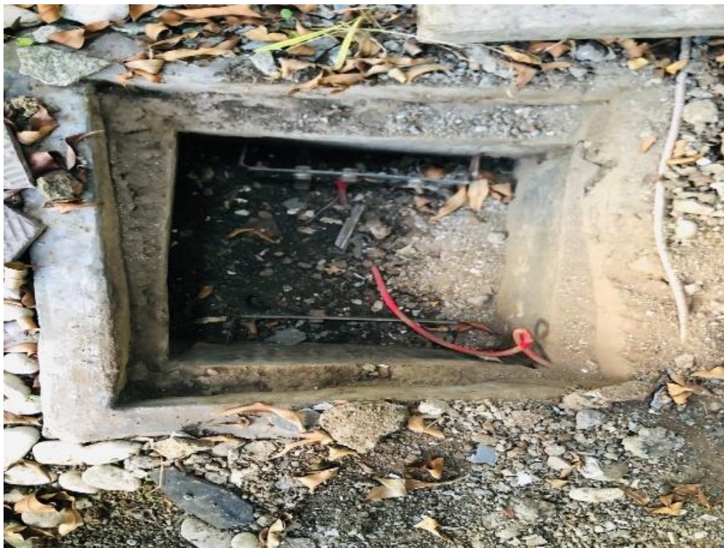
Figure 2. Condition of Grounding
