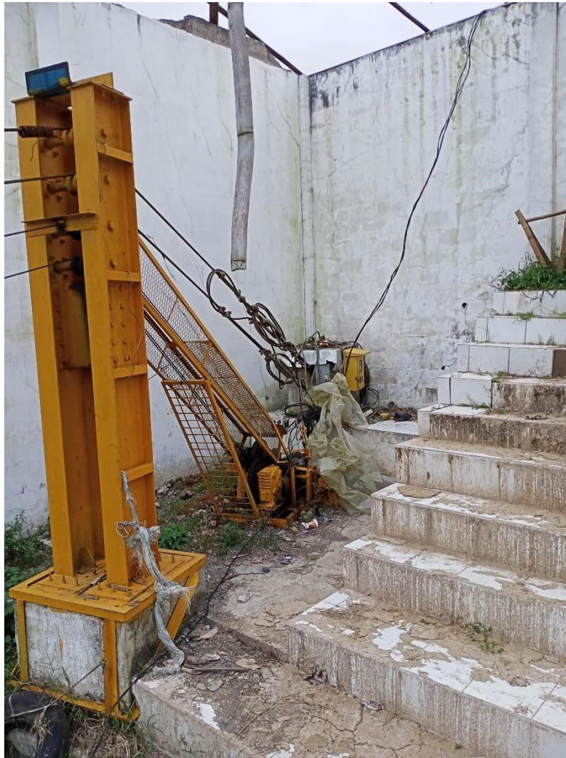
Figure 4 Support Poles and Drive Motors
