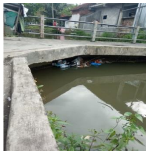
Picture 1. Trash that clogging the ditches in Petir Street
