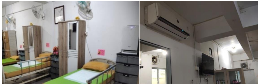
Figure 26. Artificial ventilation in an elderly room
