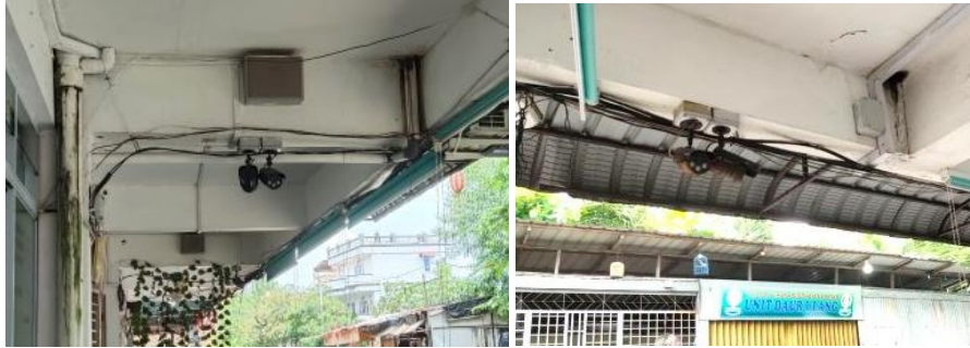
Figure 11. Installation of CCTV in the Outdoor Area of the Puri Kebajikan Nursing Home Source: Author, 2022
