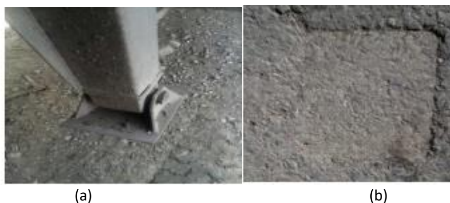
Figure 1. Deformed asphalt due to landing gear parked in before (a) and after (b) landing condition.
